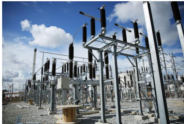
FIGURE 7—SUBSTATION BUS BARS 25
